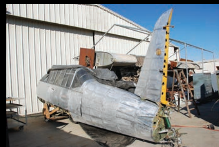
Although the fuselage surfaces looked fine from a distance, close inspection revealed corrosion in certain areas.
